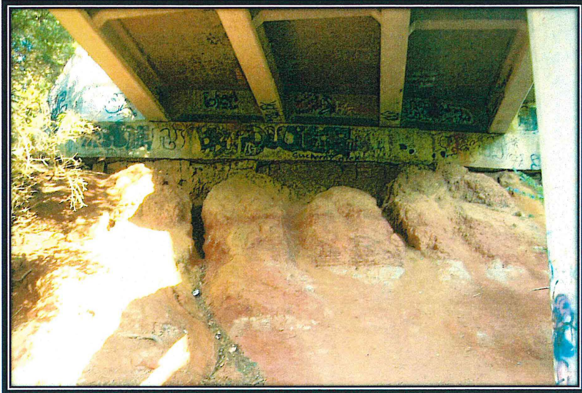
Erosion at East Abutment, West is similar
