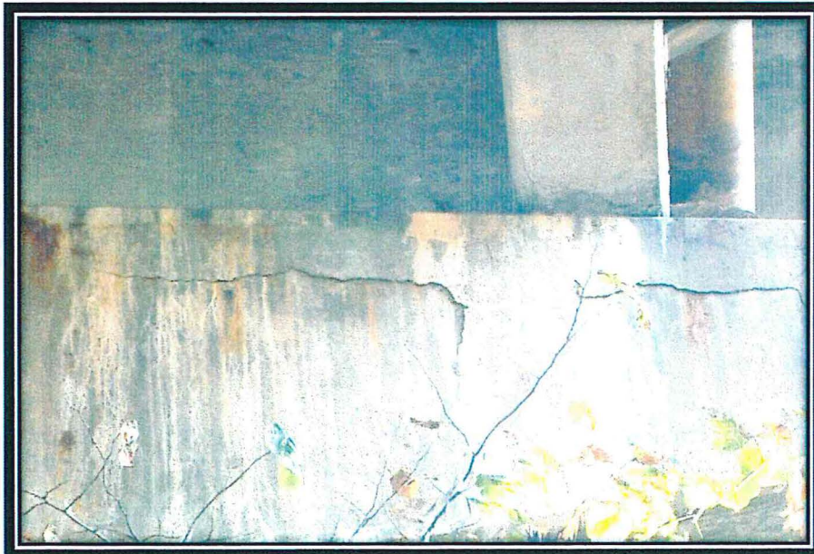
Cracks on West Pier Cap
