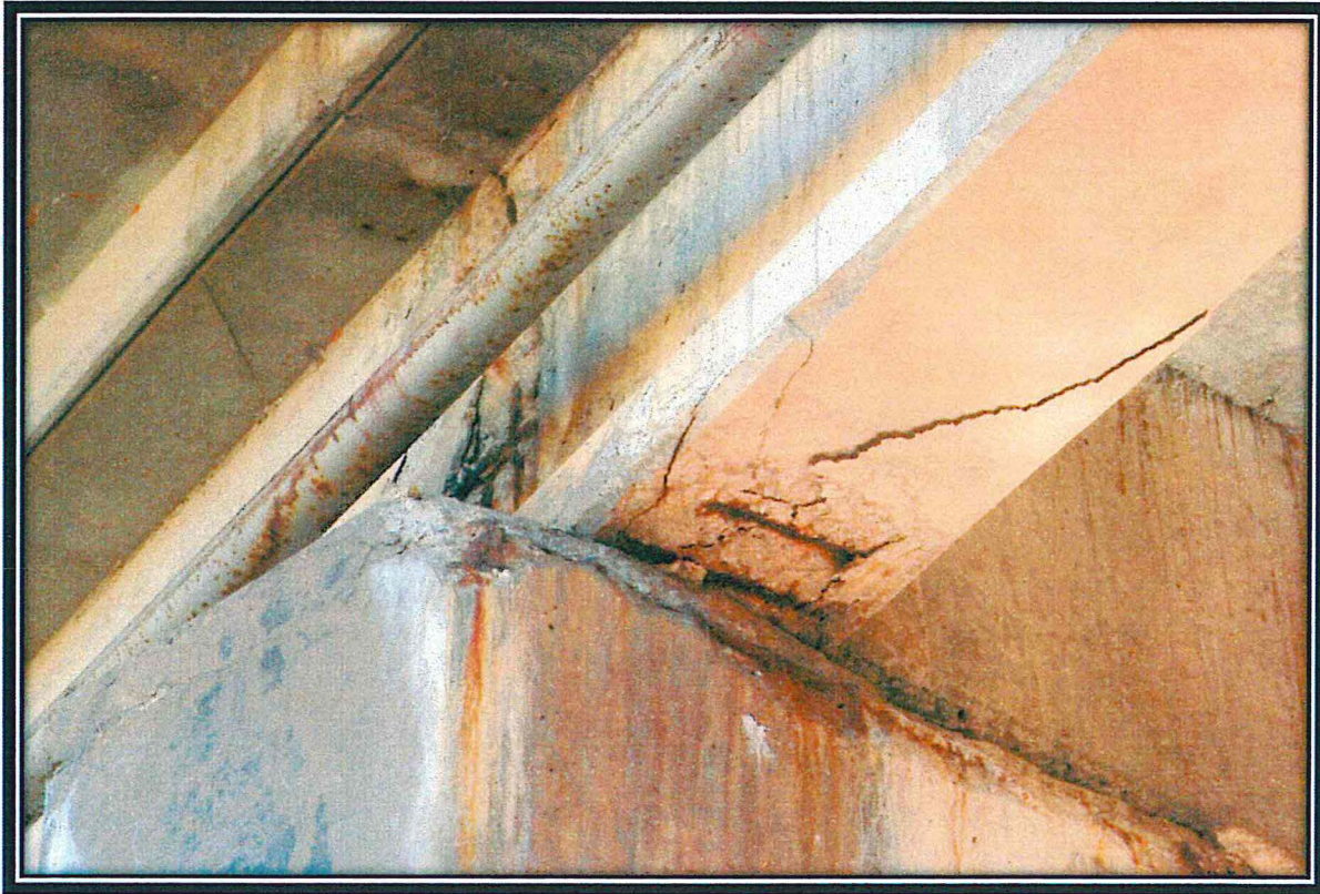
Typical Condition of Fascia Beam Ends over Piers.
