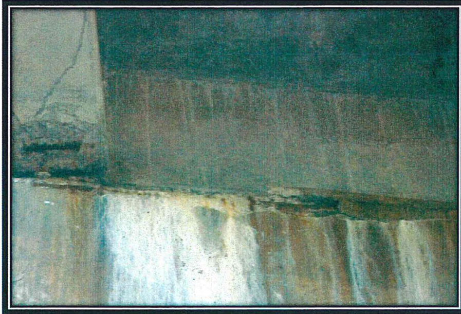
Spalling and Staining on Pier Cap
