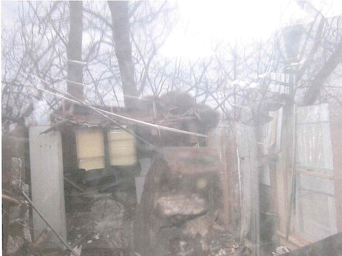
Photo 4: Inside of residence (approximately one-quarter of roof has collapsed).
