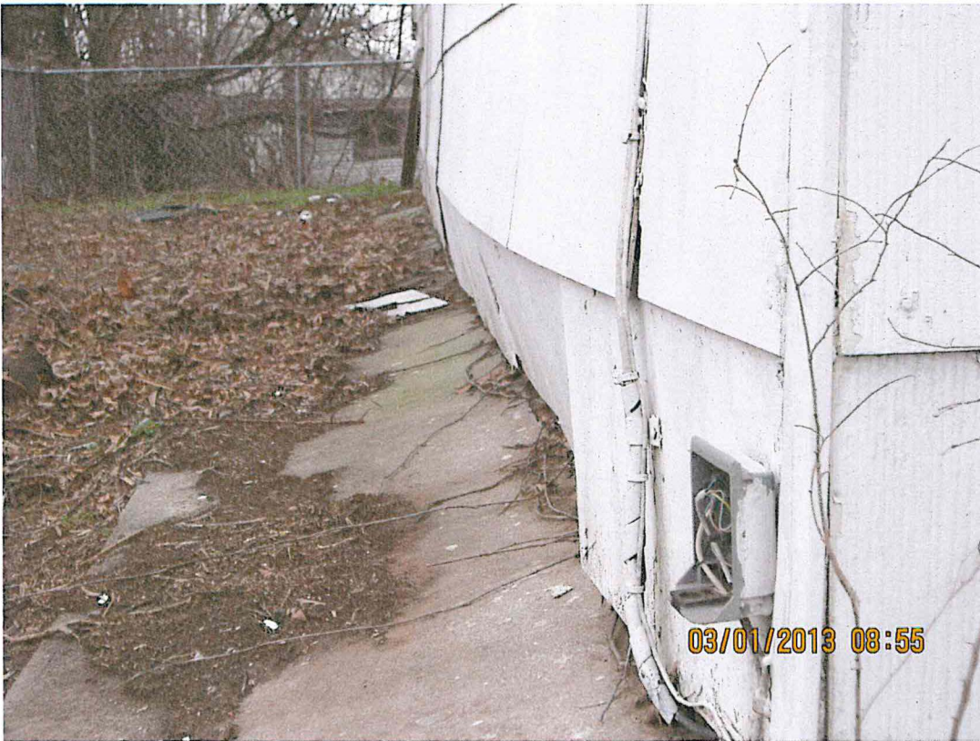
Photo 5: View of bowing foundation and exterior wall (residence).
