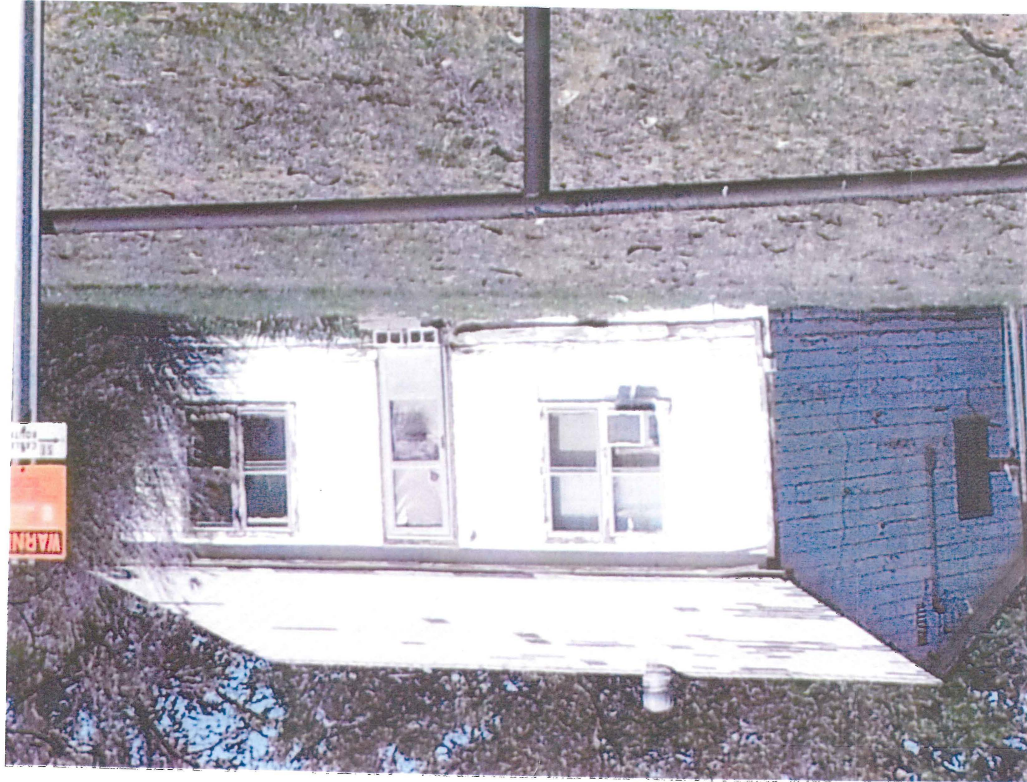
Permanent structure falling apart
