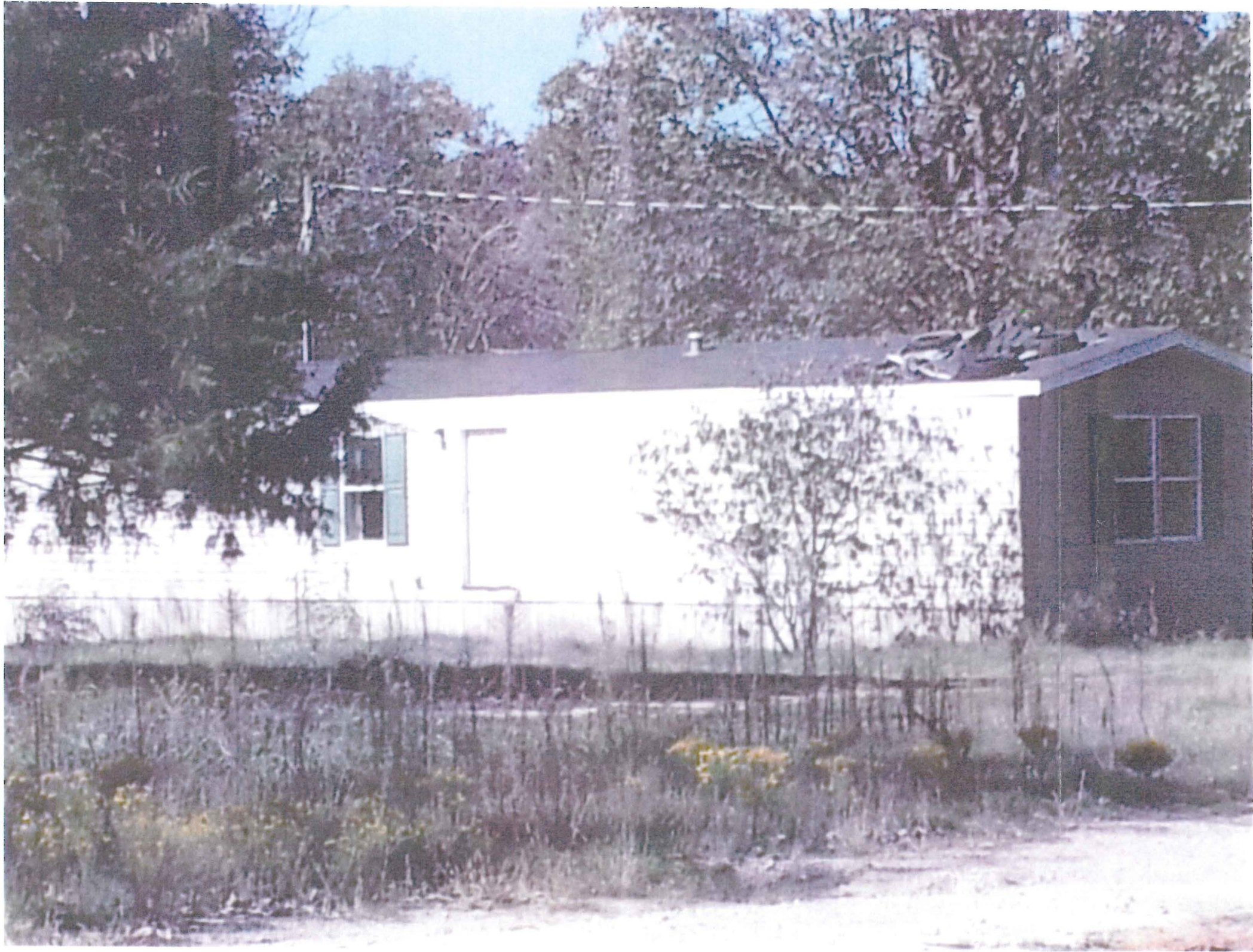
Not mowed Tires holding down tarp on roof
