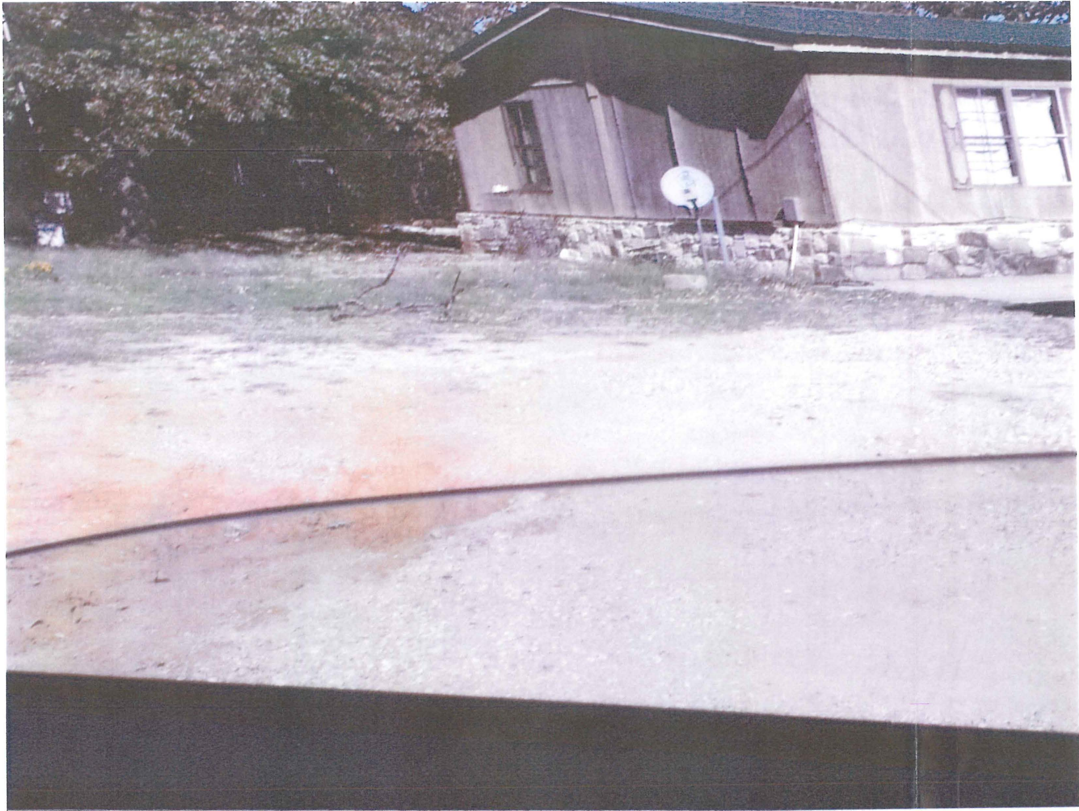
Falling apart permanently structure
