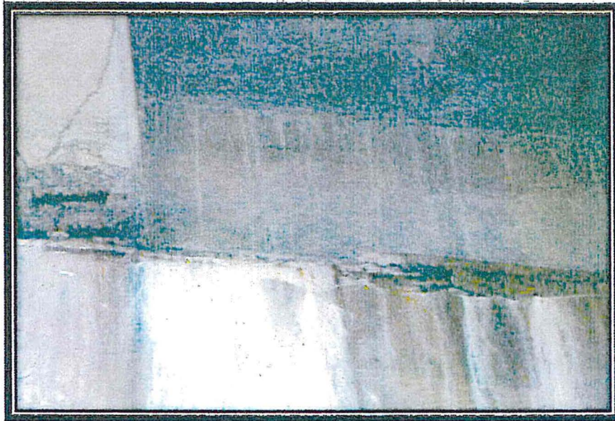
Spalling and Staining on Pier Cap
