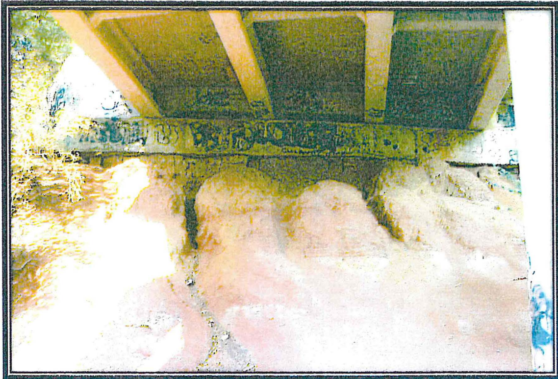
Erosion at East Abutment, West is similar
